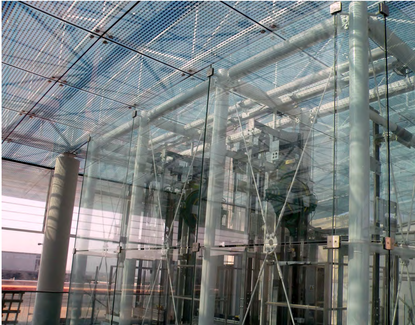
ROMA Da Vinci Business Center (INGENIUM RE srl, arch. Marco Tamino, 2011) Roof-garden e rivestimenti interni
